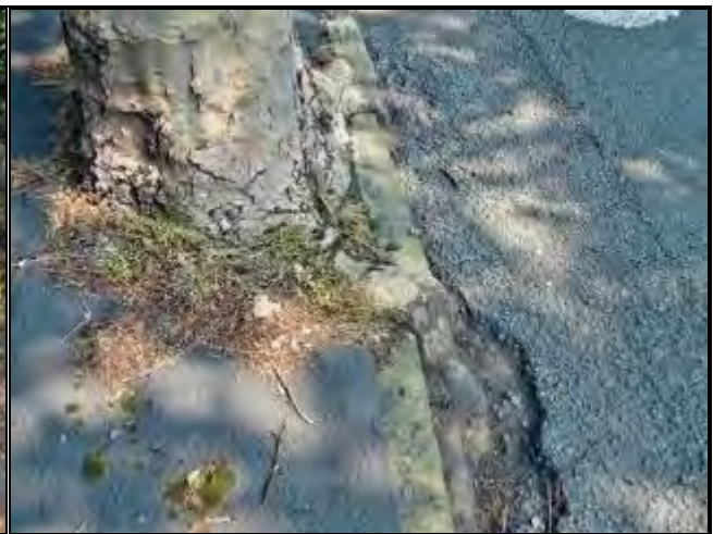
Photograph 126: Root Damage to Planetree Road
