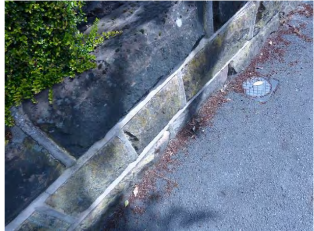
Thick pointing on Arthog Road
